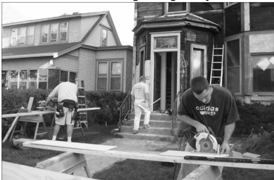
A lot of work is being done on houses throughout Dayton's Bluff. This house at 723 Margaret Street is being totally upgraded inside and out by the Dayton's Bluff Neighborhood Housing Services. This lovely Victorian home was built in 1901 by J. H. Brandhorst who built many homes in Dayton's Bluff and also lived in the neighborhood.
