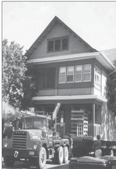
House on the Move: The Winslow Dunn house was moved from 397 Bates to 636 Bates attracting a crowd of area residents on lawnchairs.
