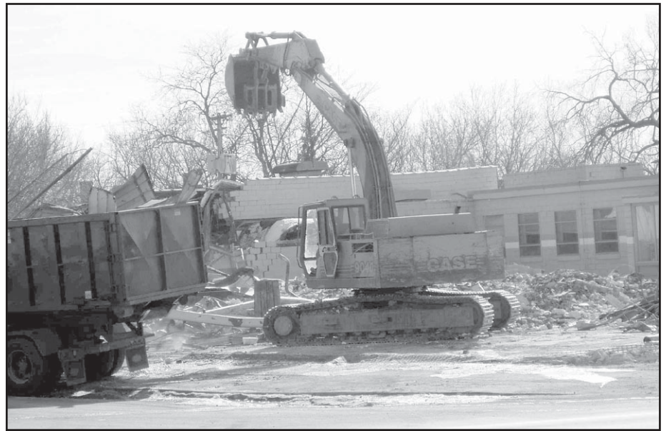
The old Hospital Linen building comes down to make way for new condos on East 7th St. at Maple. Hospital Linen moved their operations to buildings in the Hamm's Brewery complex.
